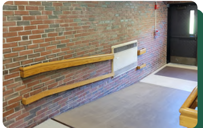
Excessive ramp slope and interrupted railing
