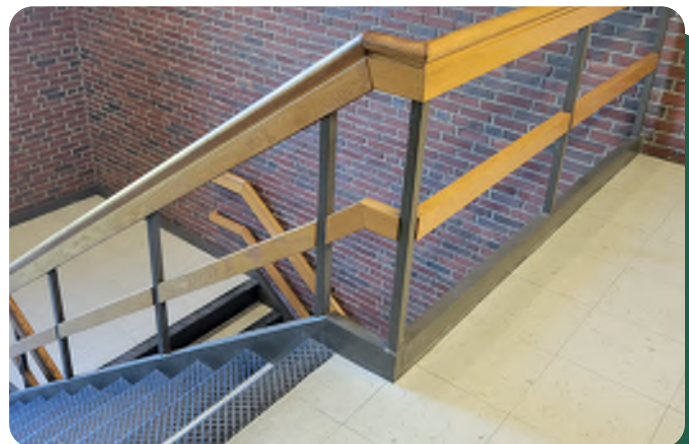
Safety stripes lacking at stair runs
