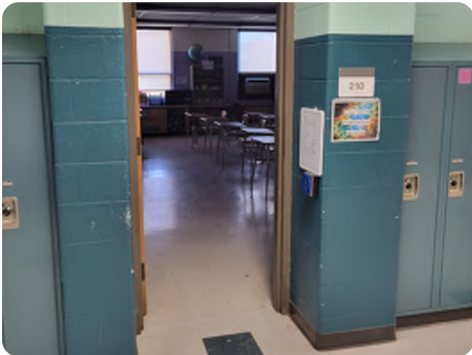
Classroom entry lacks push clearance
