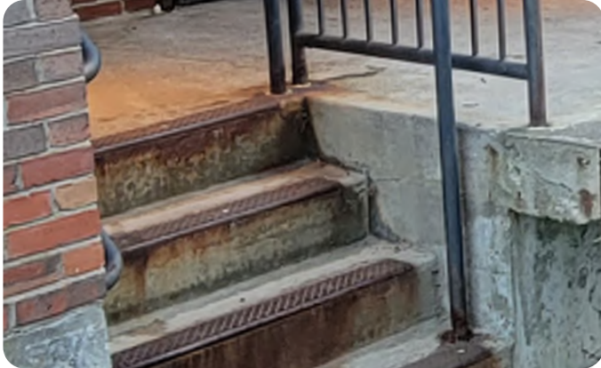
Rust at loading dock railings
