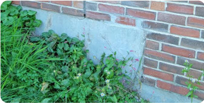
Concrete spalling at foundation
