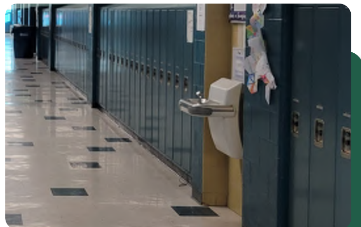
Drinking fountain projects >4" into path of travel
