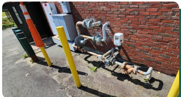
Gas Service and Meter
