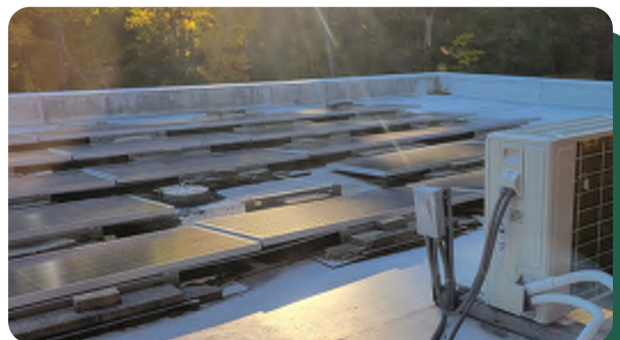
Ponding and sagging on roof
