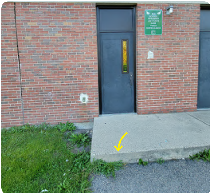
Egress utilizes a 4" step, making it inaccessible
