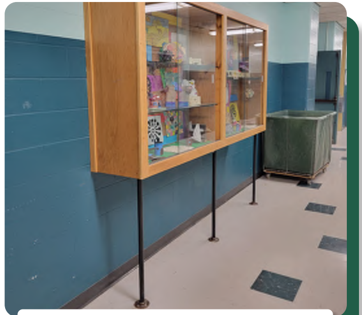
Display case protruding >12" from corridor wall
