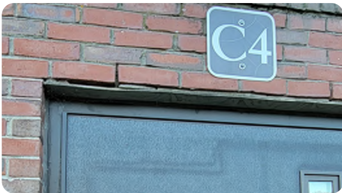
Lintel with failed sealant
