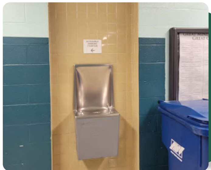
Non-accessible drinking fountain with signage
