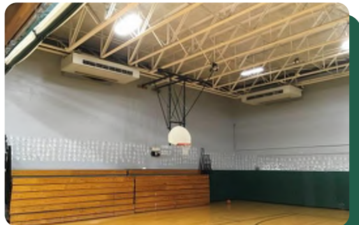
Gymnasium Horizontal Unit Ventilators
