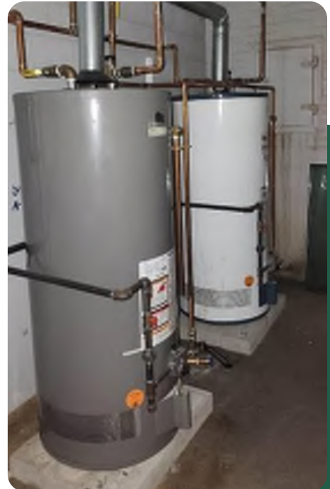
Gas Fired Water Heaters
