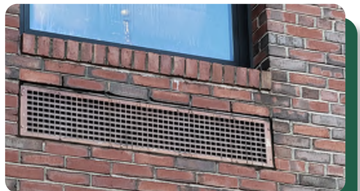
Failing sealant at grille
