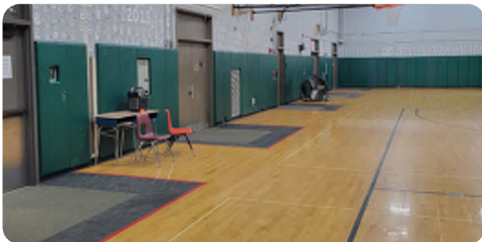
Wood athletic floor in gym with level transitions
