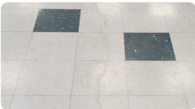
VAT in lobby with cracking
