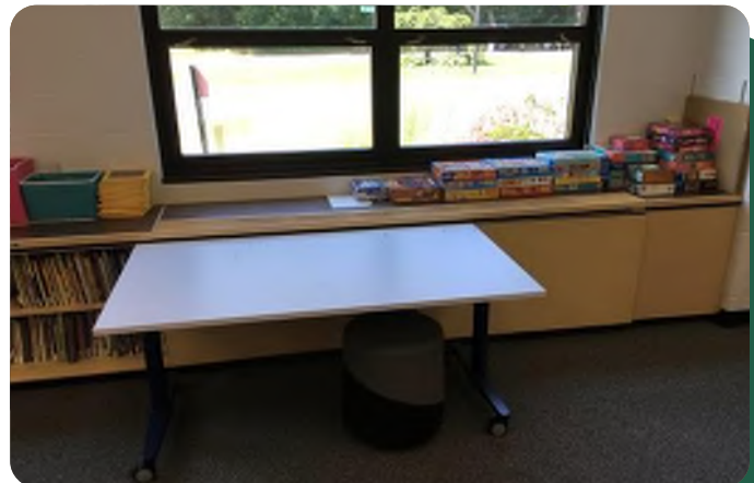
Original AAF / Herman Nelson Unit Ventilator
