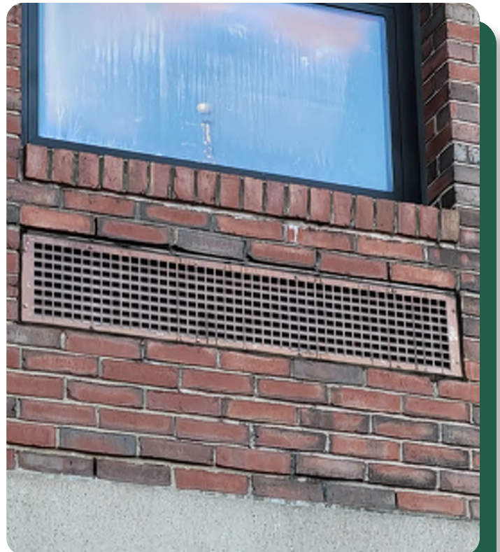
Exterior grille for unit ventilator at classroom, typ.
