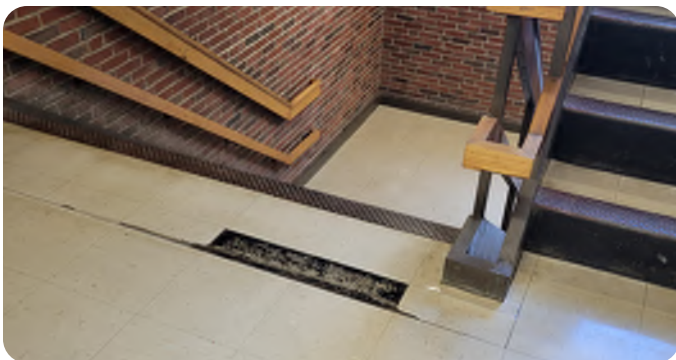
Tripping hazard at stair
