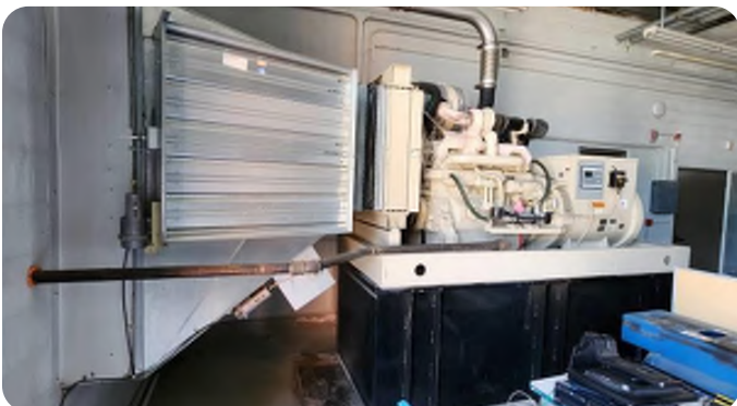
Natural Gas Generator
