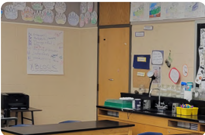
Classroom entry lacking pull clearance
