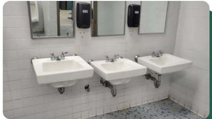
Toilet sinks are not fully accessible and lack pipe guards
