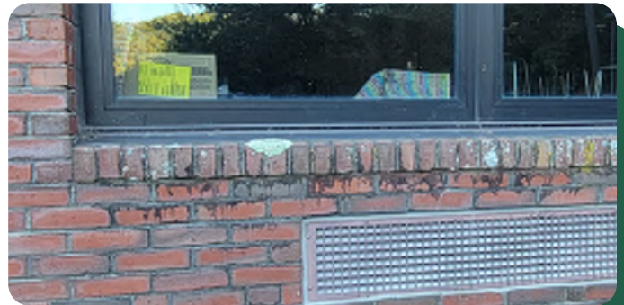
Failed mortar & moisture infiltration at rowlock sill
