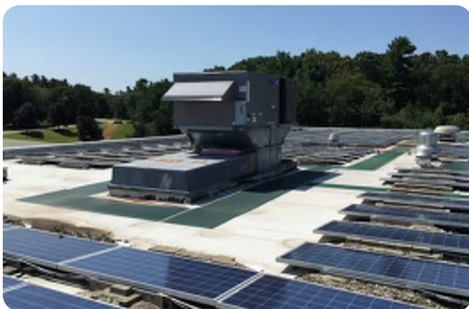
Packaged Roof Top Unit
