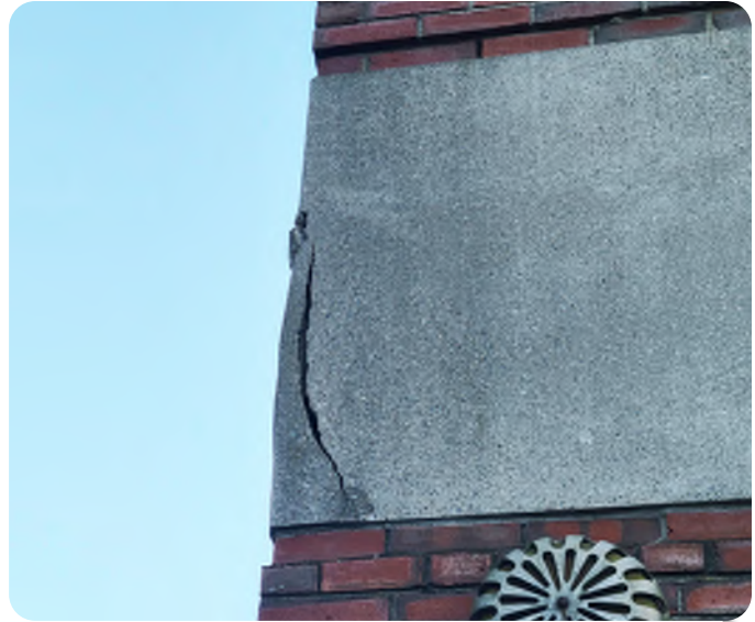
Damage to precast at southeast corner
