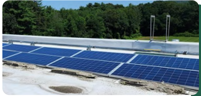
Deteriorating Concrete Pavers on Roof
