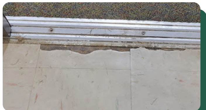
Damaged VAT at threshold
