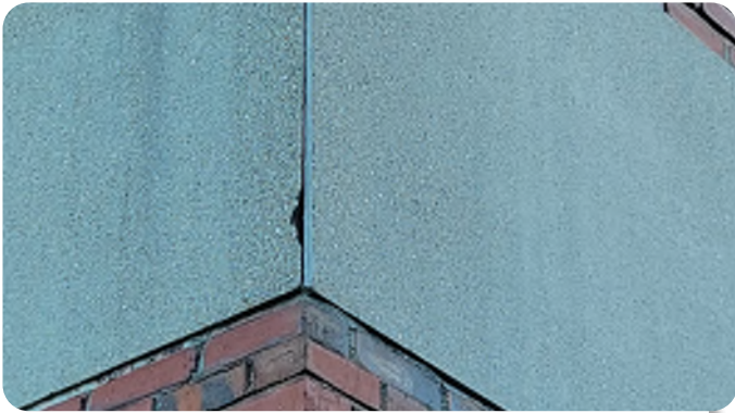
Damage at precast mitered corner
