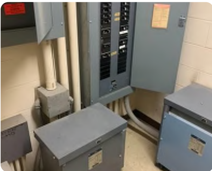
Sub Electric Room
