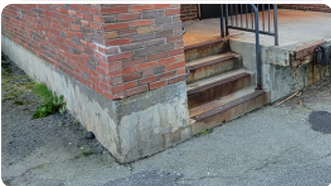
Staining on concrete
