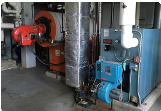
Gas fired boilers
