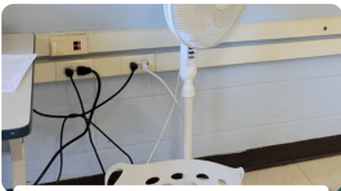
Raceway and technology ports in classroom
