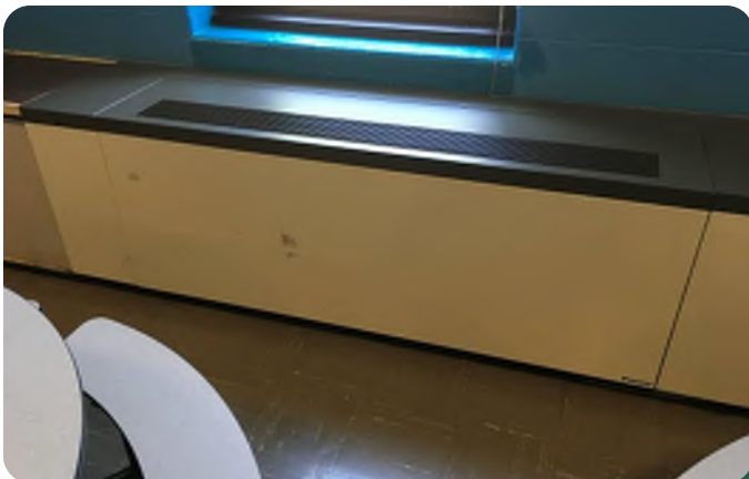
Cafetorium Unit Ventilator
