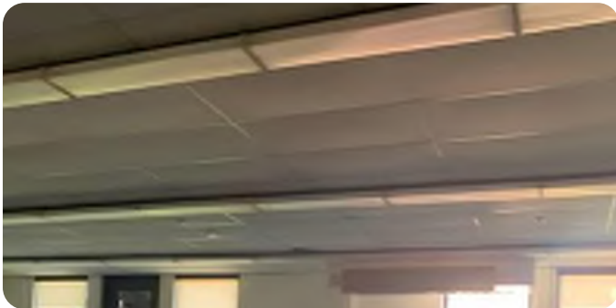
Fluorescent Lighting Fixtures
