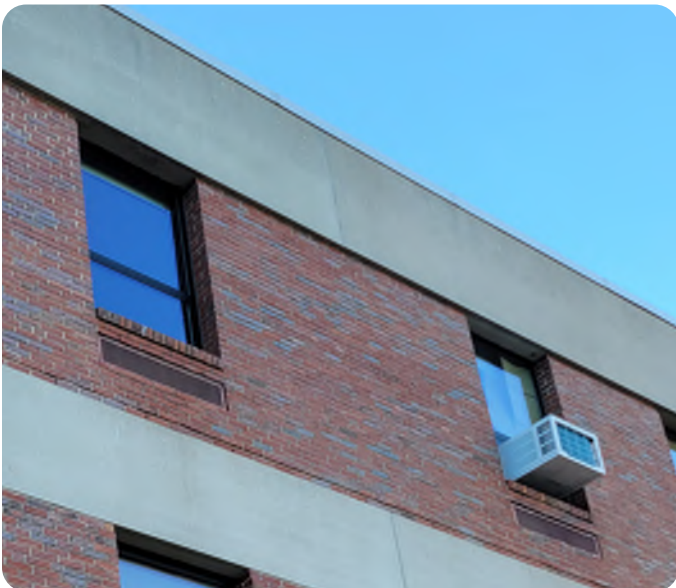
Classroom with unit air conditioner
