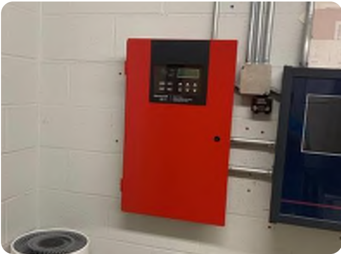
Fire Alarm Control Panel
