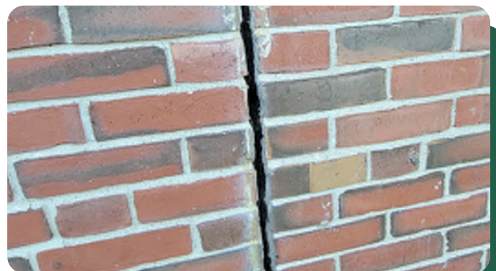
Complete failure of control joint sealant
