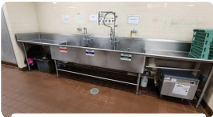
Three-pot Kitchen Sink Station
