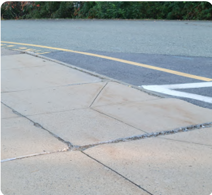
Non-compliant paving at ramp
