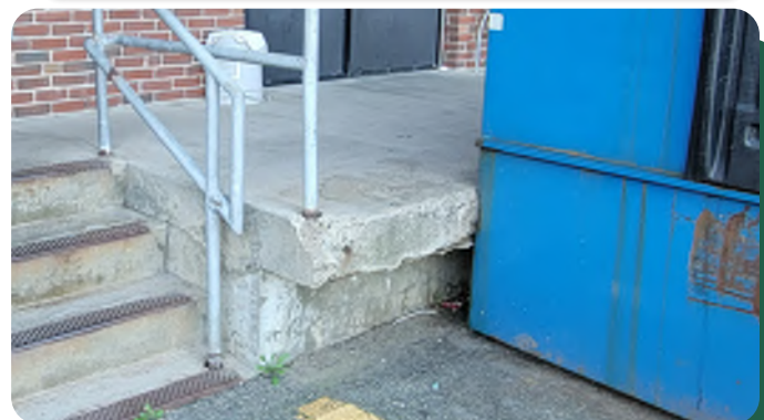
Damage at loading dock
