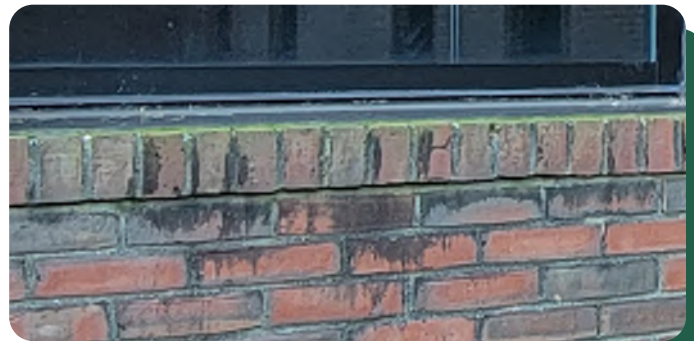
Mold and staining on bricks
