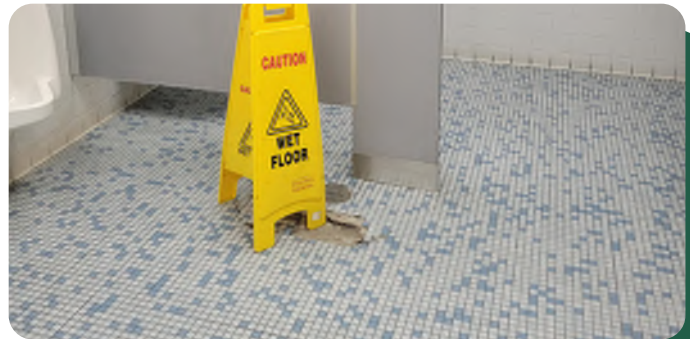
Damaged floor tile in toilet room
