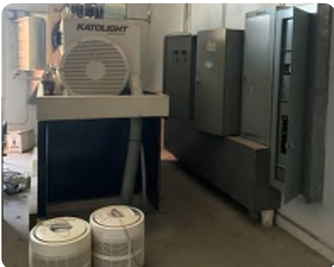
Generator, Emergency Panel, and ATS
