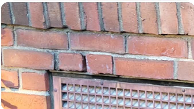
Example of bricks that require repointing
