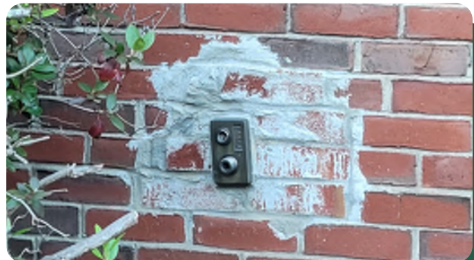
Patch / repair requiring remediation
