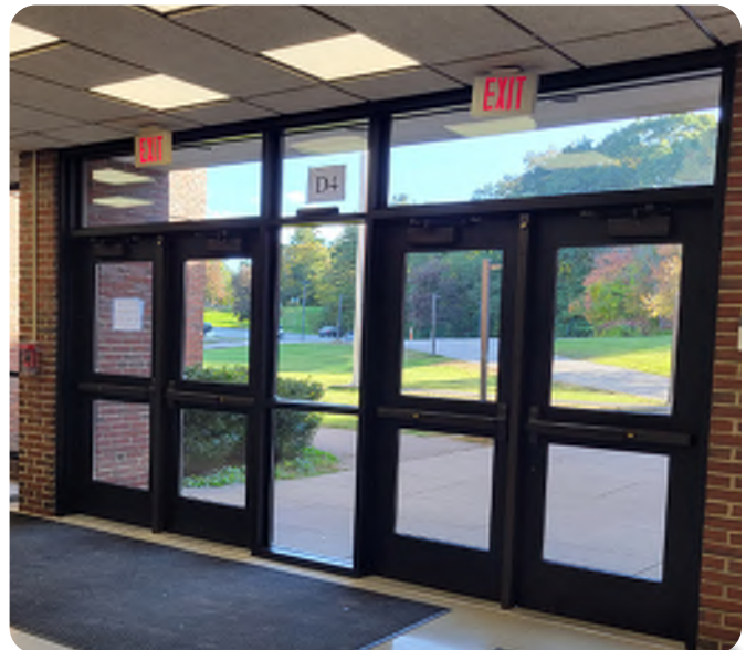
Building entrance with no vestibule
