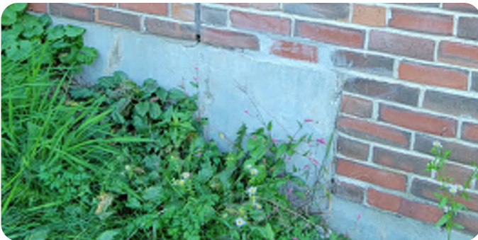
Concrete spalling at foundation
