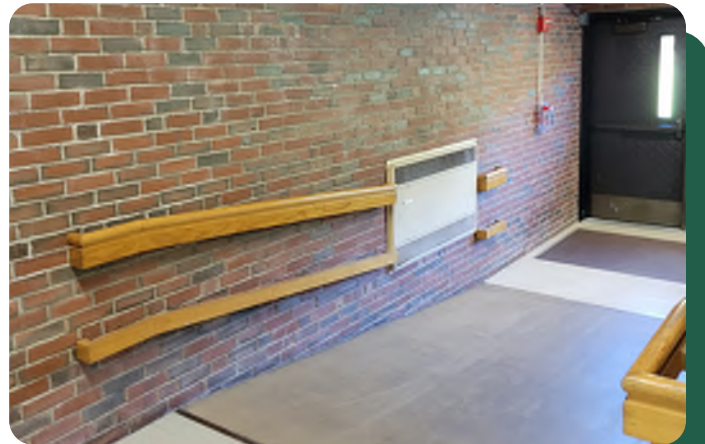
Excessive ramp slope and interrupted railing
