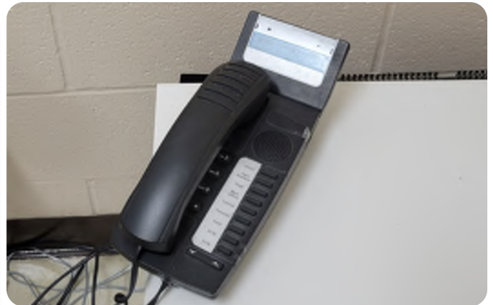
Typical telephone unit in classroom
