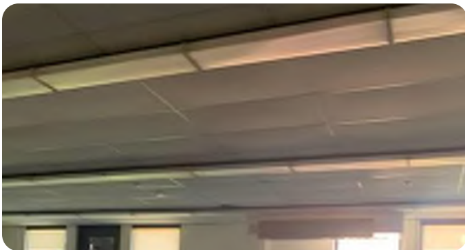
Fluorescent Lighting Fixtures
