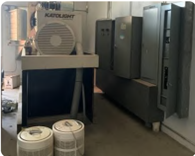
Generator, Emergency Panel, and ATS
