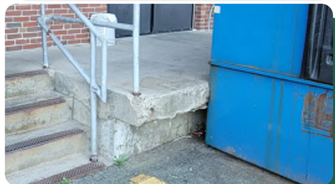
Damage at loading dock
