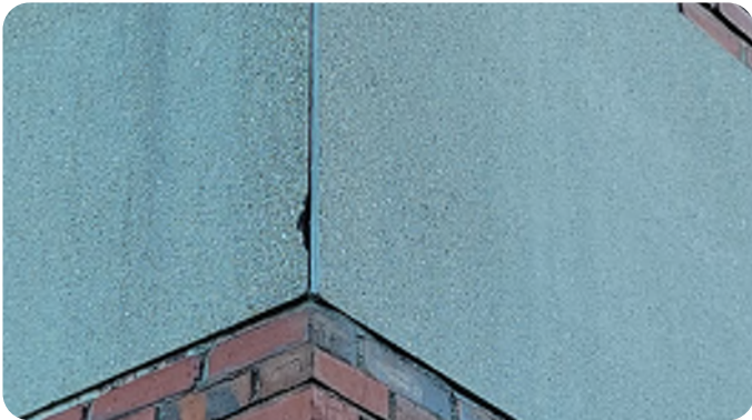
Damage at precast mitered corner
