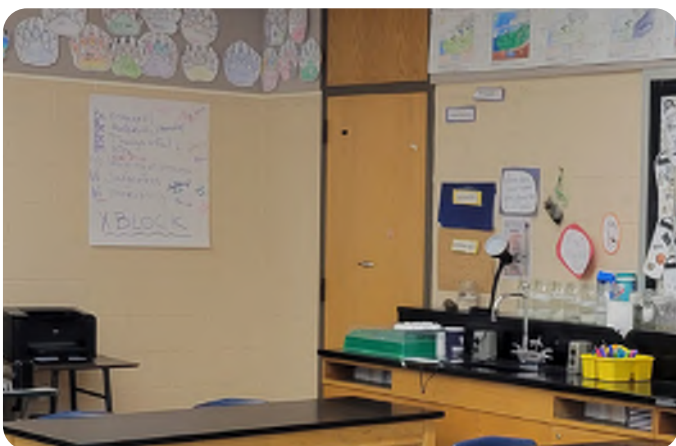
Classroom entry lacking pull clearance
