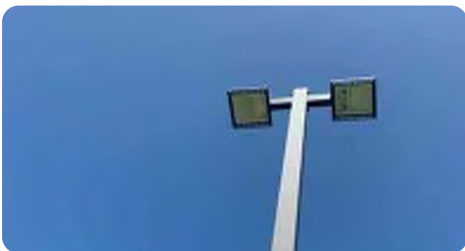
Pole Site Lighting Fixture
