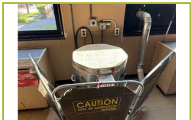
Photograph #36: Kiln in art room.
