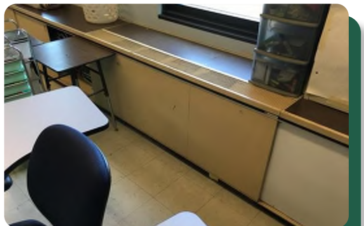
Typical Classroom Unit Ventilator
