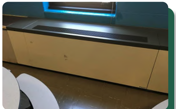
Cafetorium Unit Ventilator
