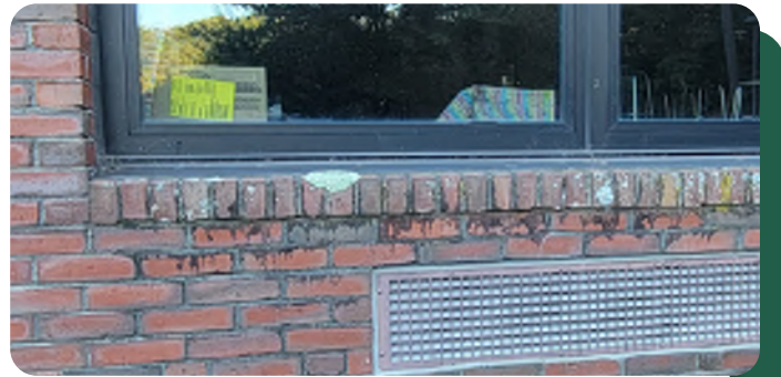
Failed mortar & moisture infiltration at rowlock sill
