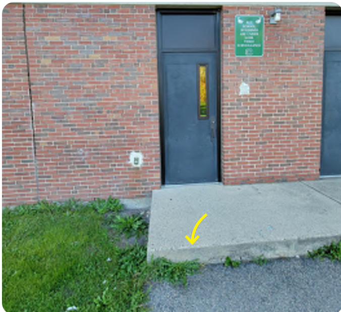
Egress utilizes a 4" step, making it inaccessible
