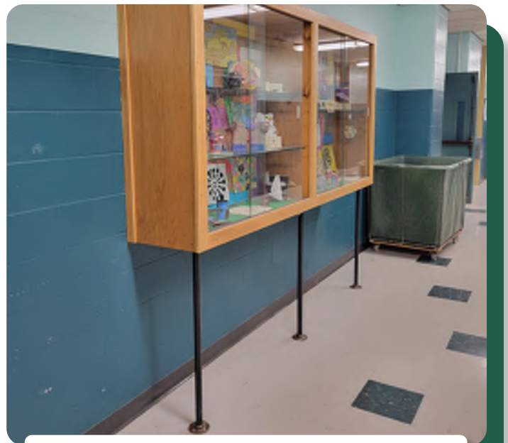
Display case protruding >12" from corridor wall
