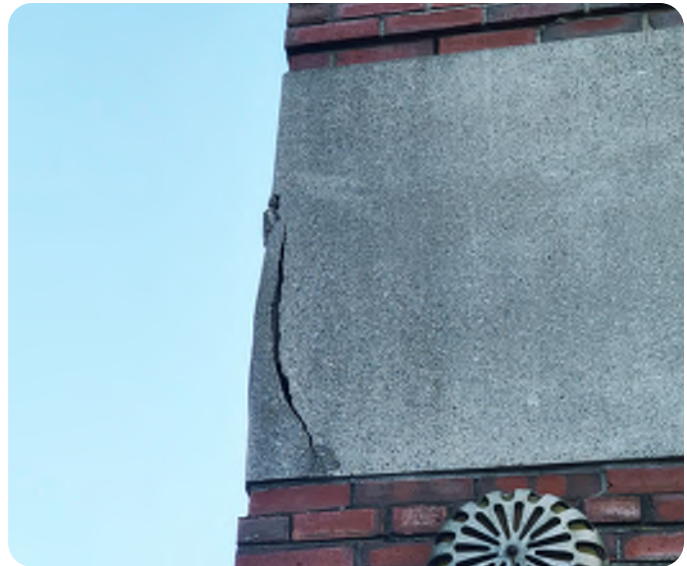
Damage to precast at southeast corner
