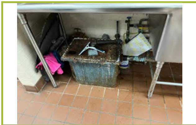
Photograph #17: Grease trap.
