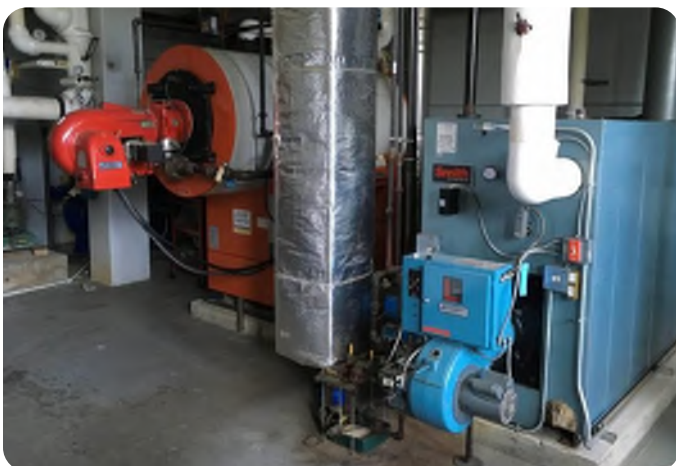
Gas fired boilers
