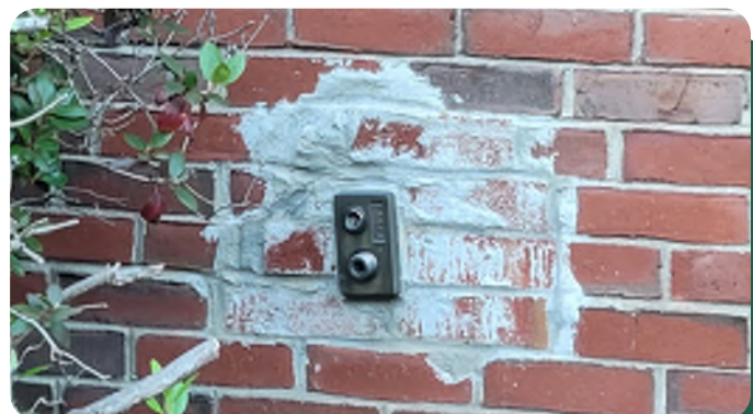
Patch/repair requiring remediation
