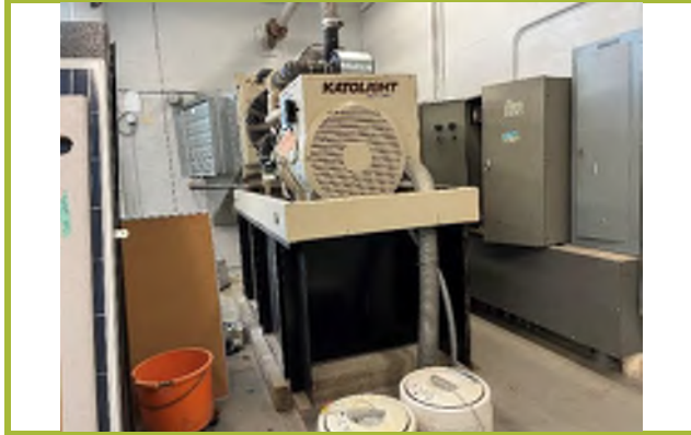
Photograph #25: Emergency generator.
