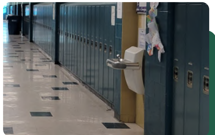
Drinking fountain projects >4" into path of travel
