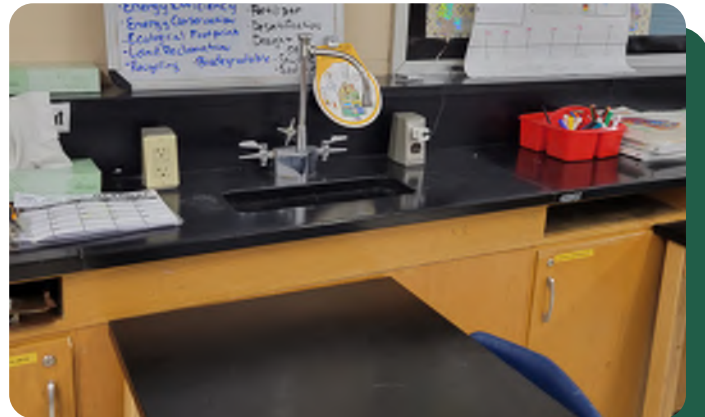
Science sinks that do not meet accessibility req's
