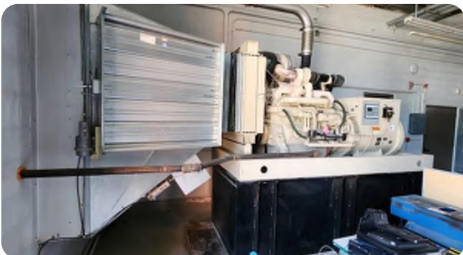
Natural Gas Generator
