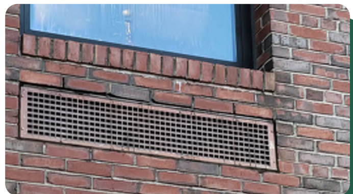
Failing sealant at grille
