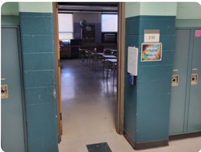
Classroom entry lacks push clearance
