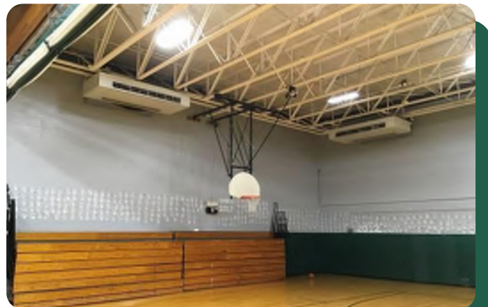
Gymnasium Horizontal Unit Ventilators
