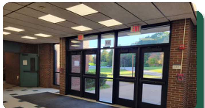
Lack of door operators at main building entrance
