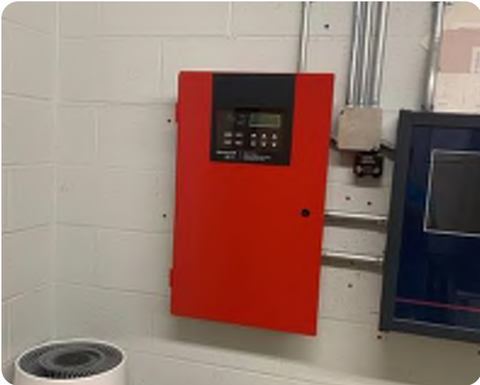
Fire Alarm Control Panel
