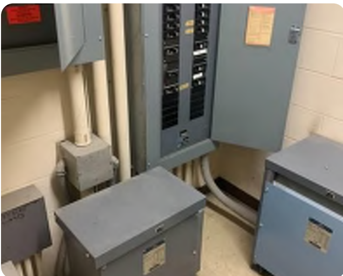
Sub Electric Room
