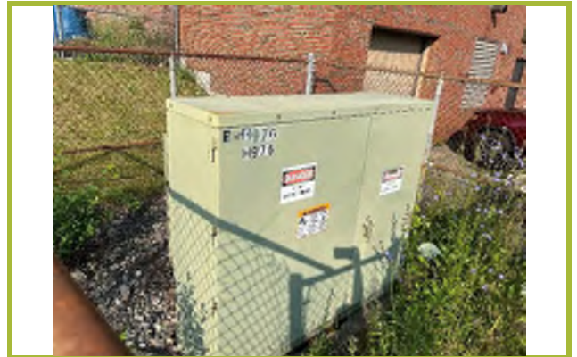
Photograph #4: Pad-mounted transformer.
