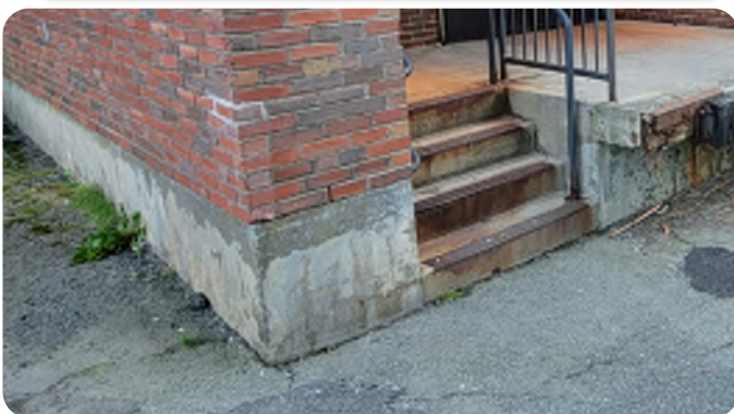
Staining on concrete
