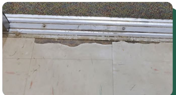
Damaged VAT at threshold
