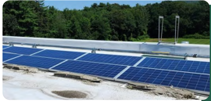
Deteriorating Concrete Pavers on Roof
