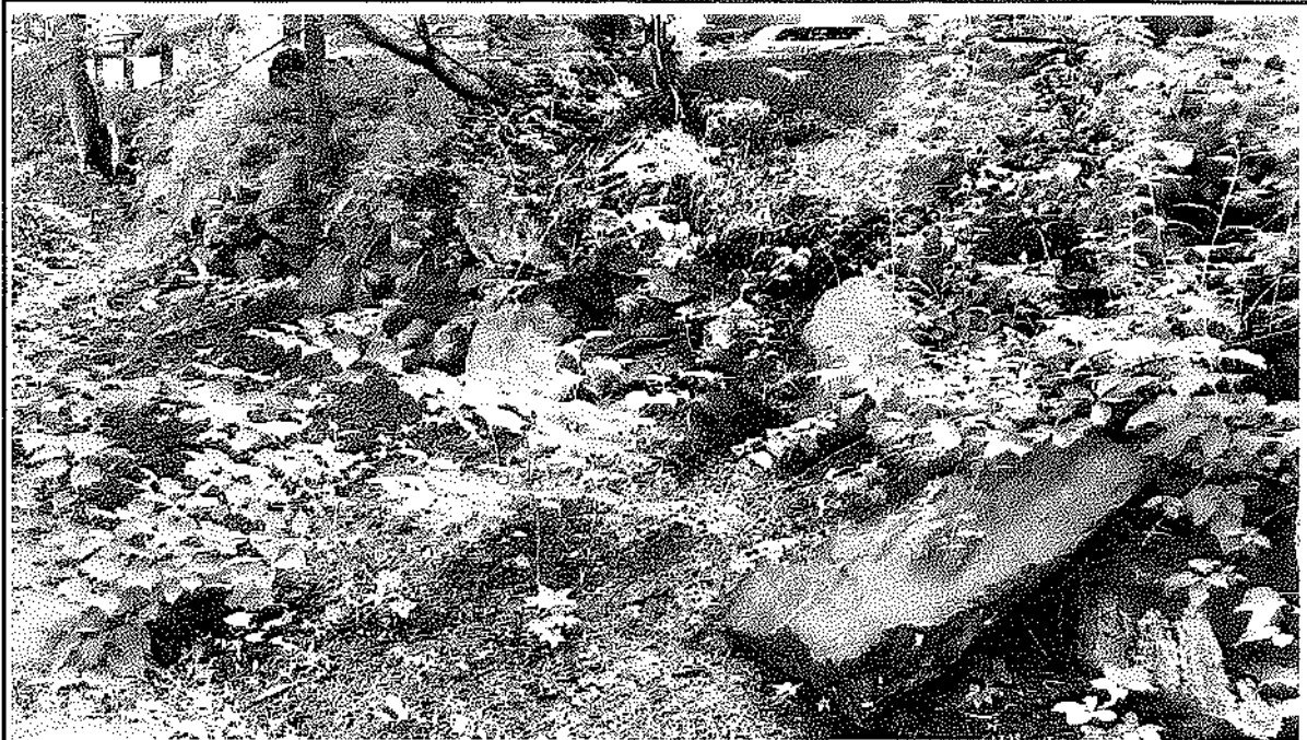
Photo taken July 19, 2021 of downstream wall west of culvert, looking southeast, showing dislodged stone and bulging/misaligned wall.
