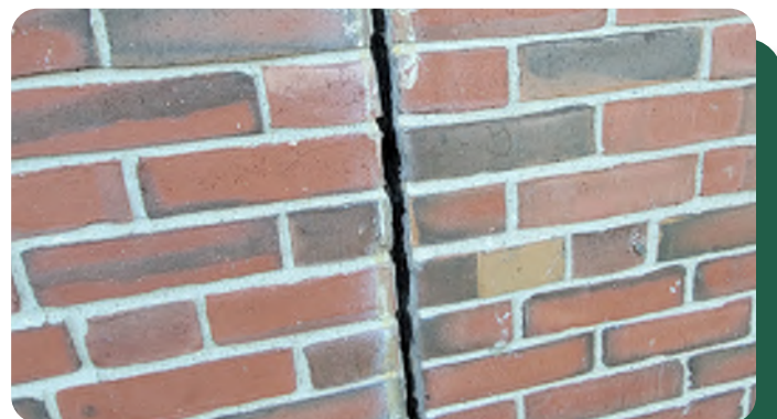
Complete failure of control joint sealant
