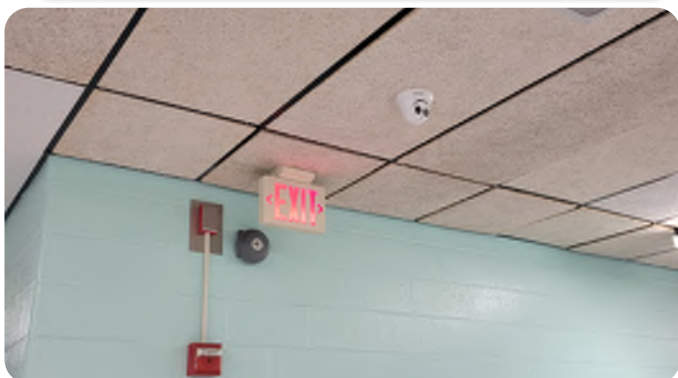
Corridor security camera
