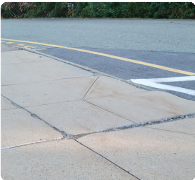
Non-compliant paving at ramp
