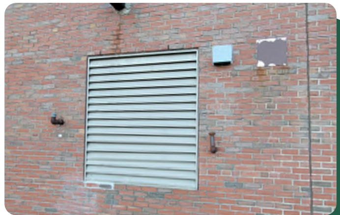
Mechanical louver in good condition
