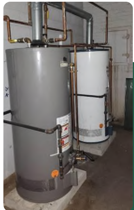
Gas Fired Water Heaters
