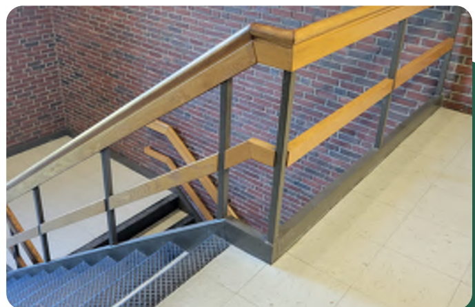
Safety stripes lacking at stair runs
