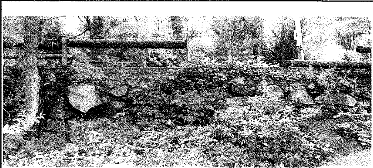
Photo taken July 19, 2021 of downstream wall west of culvert, looking upstream (southeast), showing voids between stones
