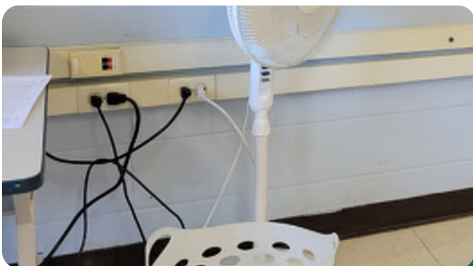
Raceway and technology ports in classroom
