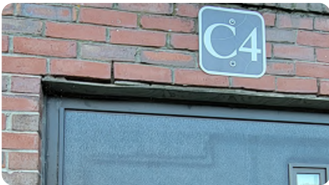
Lintel with failed sealant
