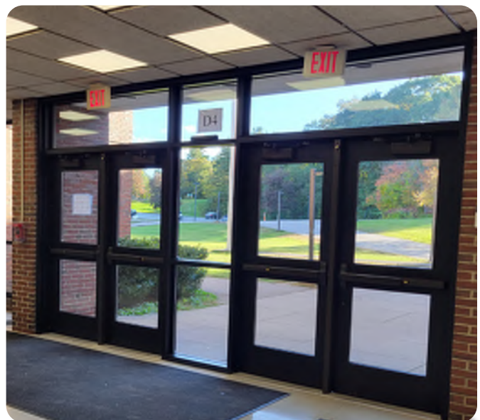
Building entrance with no vestibule
