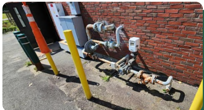
Gas Service and Meter
