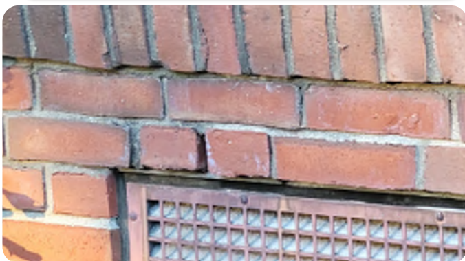
Example of bricks that require repointing
