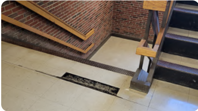
Tripping hazard at stair
