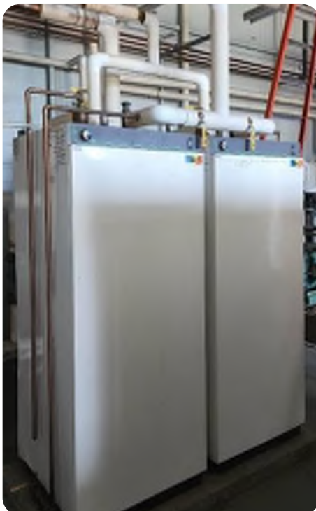
Indirect Water Heaters
