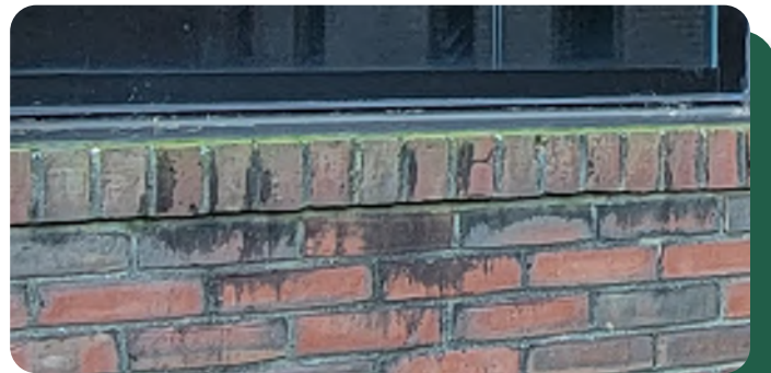
Mold and staining on bricks
