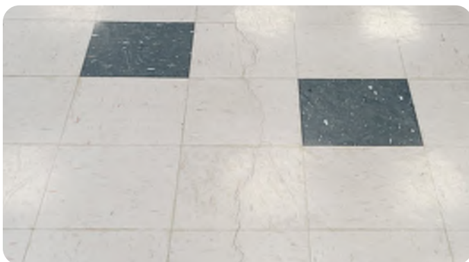
VAT in lobby with cracking
