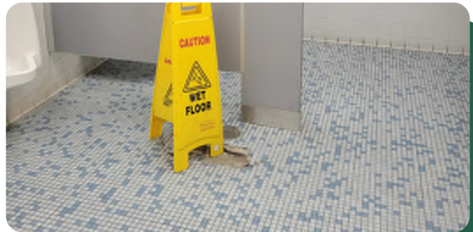
Damaged floor tile in toilet room
