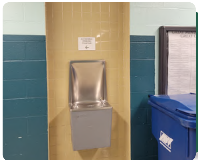
Non-accessible drinking fountain with signage
