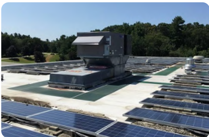
Packaged Roof Top Unit
