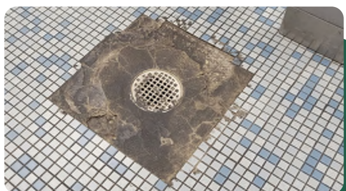
Damaged tile at toilet room drain
